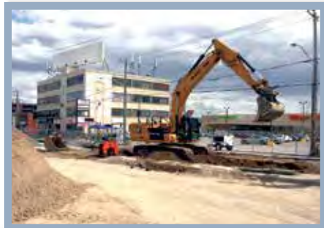
Laval and other cities need a new deal from the Quebec government given the skyrocketing costs for important infrastructure work like this water infrastructure project in 2021 near the corner of Curé Labelle and Notre Dame in Chomedey. (Photo: Martin C. Barry, Newsfirst Multimedia)
