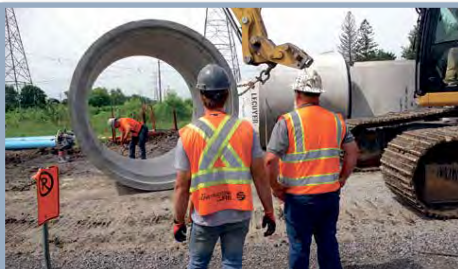
Among the stormwater drain infrastructure projects being undertaken by Laval this year is the modernization of systems in the Vimont district to reduce the risk of backups and stormwater flooding. (Photo: Martin C. Barry, Laval News)
