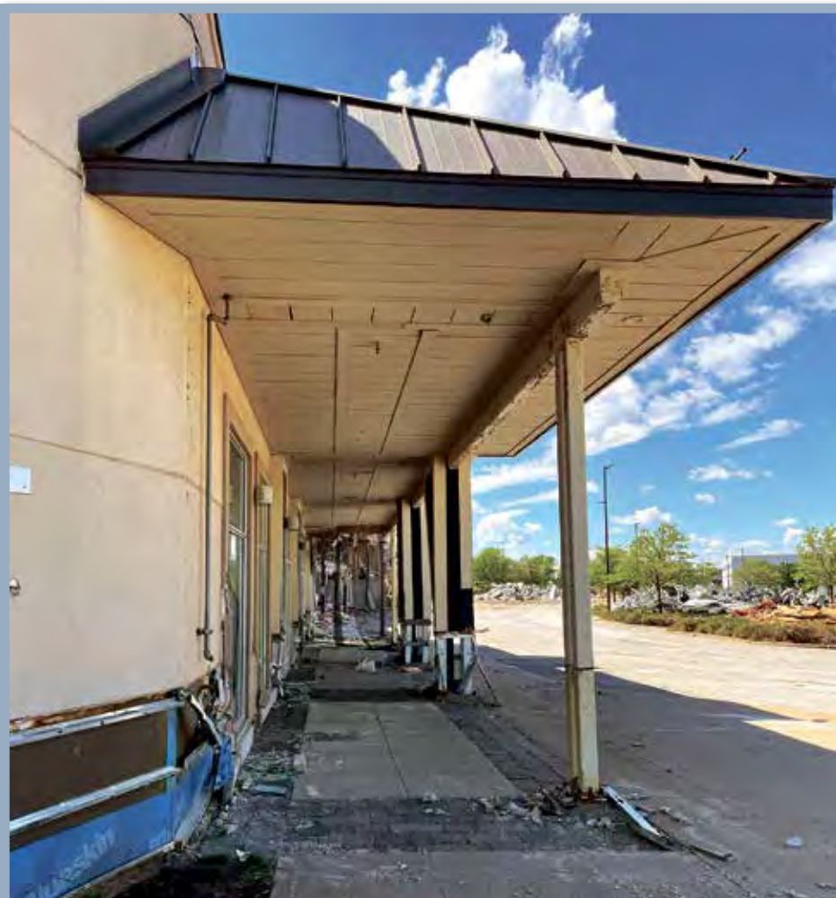
Demolition got underway last week on vacant former discount retail outlets like this one at the northern end of the Méga Centre Notre-Dame in Sainte-Dorothée in preparation for the development of new infrastructure to reinforce Laval's supply-chain and logistics corridor.
